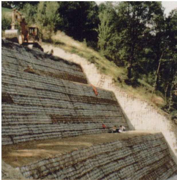
Figure 3. View of the reinforced slope in Montone at completion of construction (Coluzzi et al. 1997)
