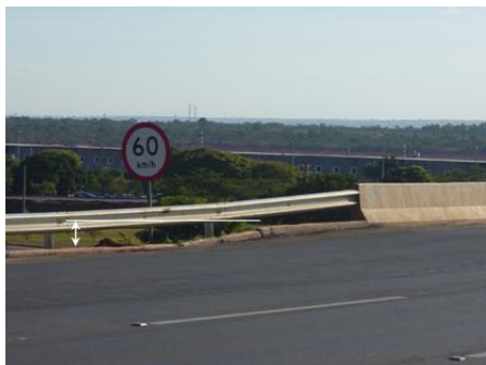
Figure 1. Excessive abutment settlement due to foundation soil structural collapse.
