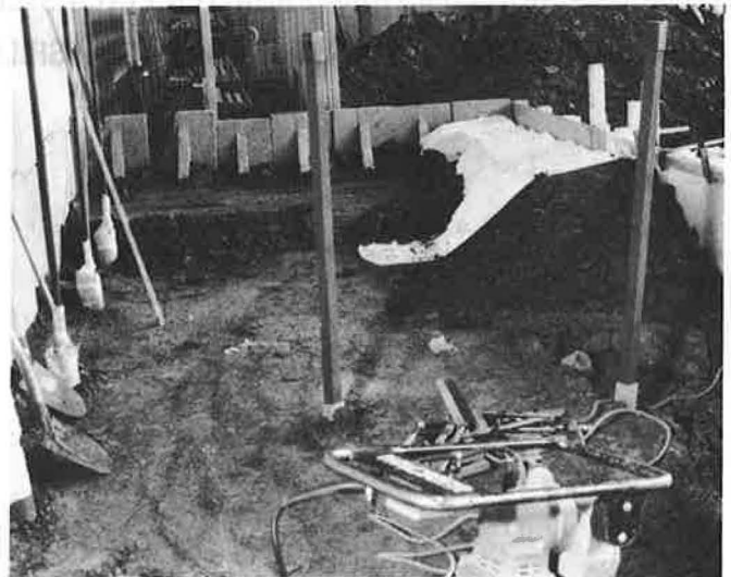
Fig. 3 - Detail of wall construction showing the fabric folded back into the construction
