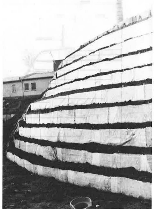
Fig. 10 View of the external wall of a very steep slope during the state of construction
