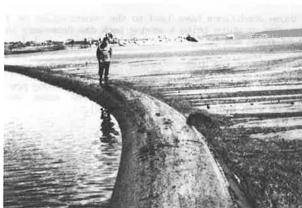
photo 1 : Construction of a temporary dike on liquid mud to provide a hydraulic fill deck
