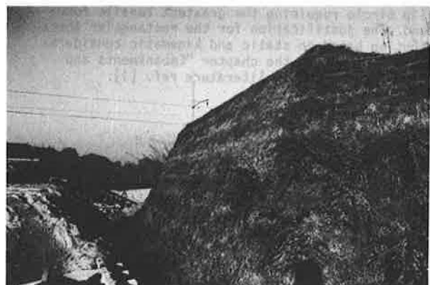
Photo no. 3: Grassed and mowed reinforcing structure 4 months after completion Location: Herisau, Switzerland altitude approx. 800 m a.s.l. SW exposition of main slope.
