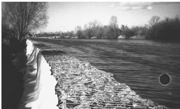
Figure 12. Valenciennes : Two-layer filtration system in contact with gabions along the Trith canal.
