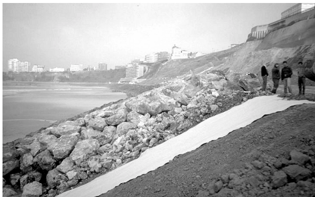
Figure 9. Biarritz - Côte de Basques : Two-layer geotextile filtration system covered by two layers of secondary
