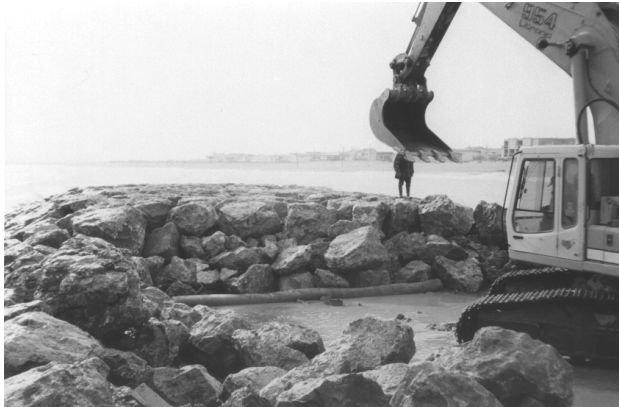
Figure 10. Valras-Plage : placing of rockfill on the filtration system (rolled in the front of the job zone due to the very small working area).
