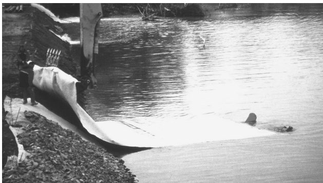
Figure 14. Hérault river : installation of the ballasted two-layer filtration system by a diver.
