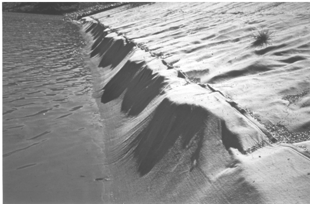
Figure 3. Valcros : Step-like deterioration of the upstream facing under the "geotextile only" test zone.
