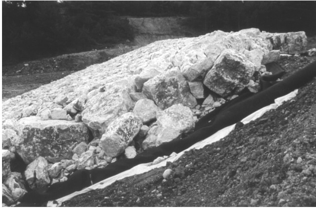
Figure 7. Salles-sur-Verdon : rip-rap laid on the geotextiles for protection (black) and for filtration (grey).
