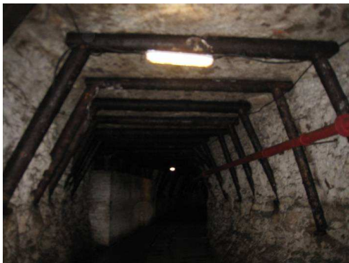
Figure 2. Oil shale mine similar type under the building site.
