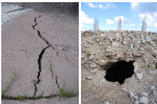
Figure 3. Cracks due to sinkhole and sinkhole on the site
