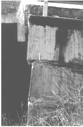
Figure 11. Rotation of wall face and facing units in Case History 4.
