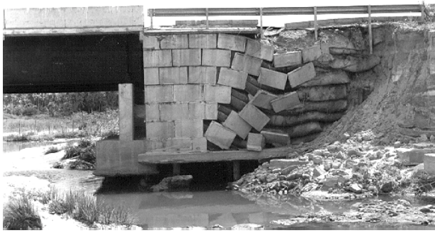
Figure 9. Facing units collapse in Case History 2.
