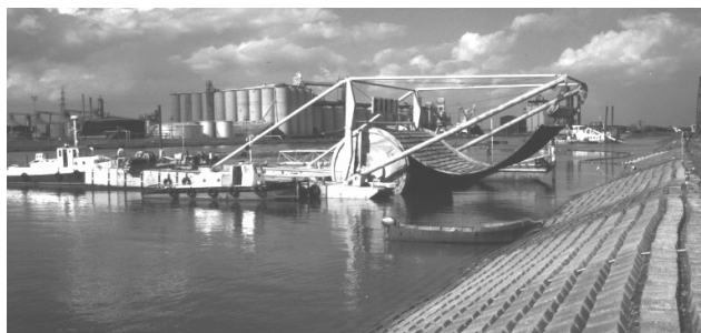
Figure 7 : Ravenna harbor. Installation of the composite on the slope with floating cylinder
