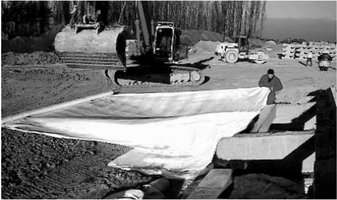
Figure 4. Geotextile being pulled up to the concrete facing element prior to placing beneath the concrete cross beam.
