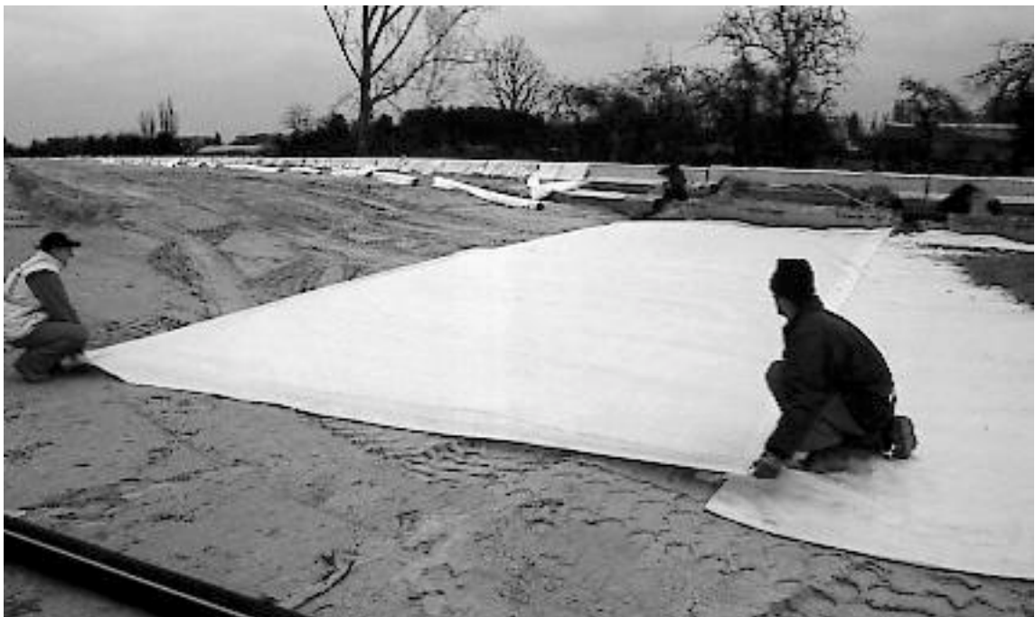
Figure 5. Reinforcing geotextile is pulled out to the precise pre-measured length as supplied to site from the factory.
