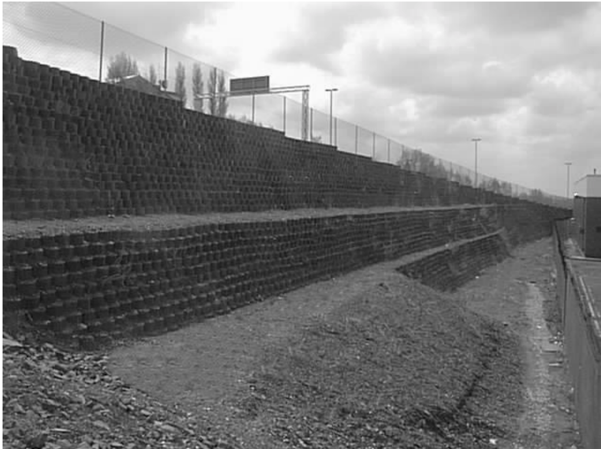
Figure 14. A 7 m high geocell retaining wall from a highway construction site in the U.K. No vegetation soon after construction.
