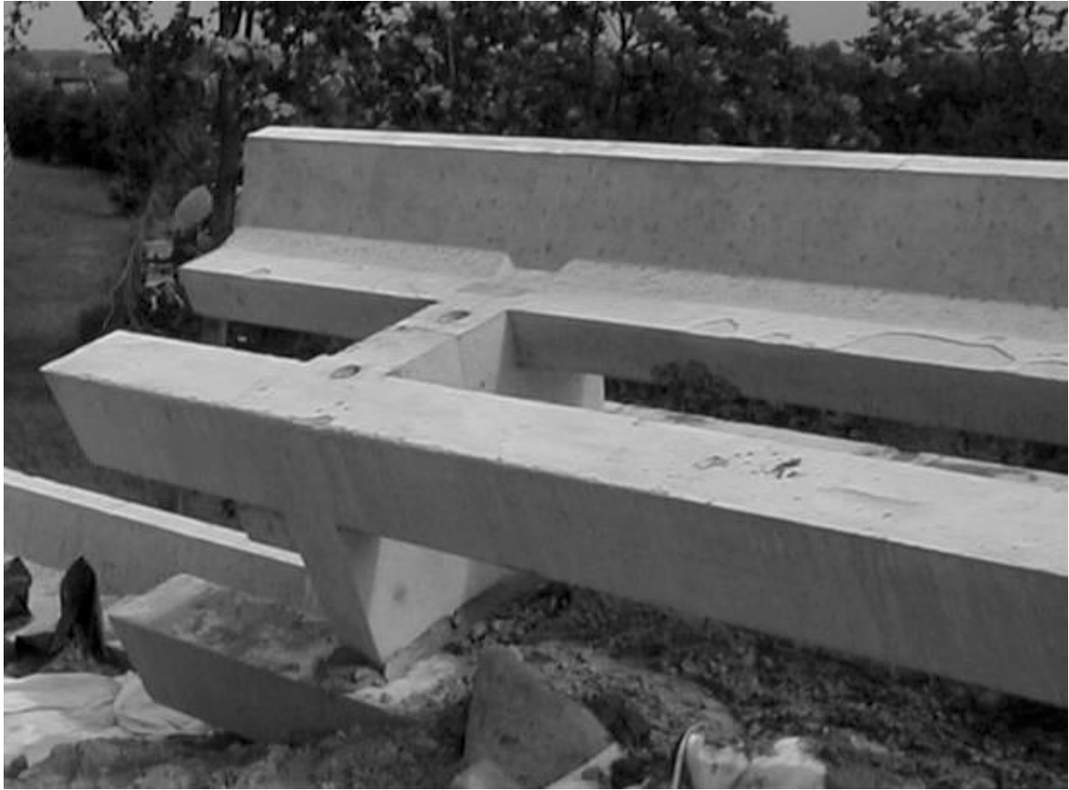
Figure 3. An empty concrete facing element viewed from inside the noise barrier. Note textiles at the base which have been wrapped round the element beneath.
