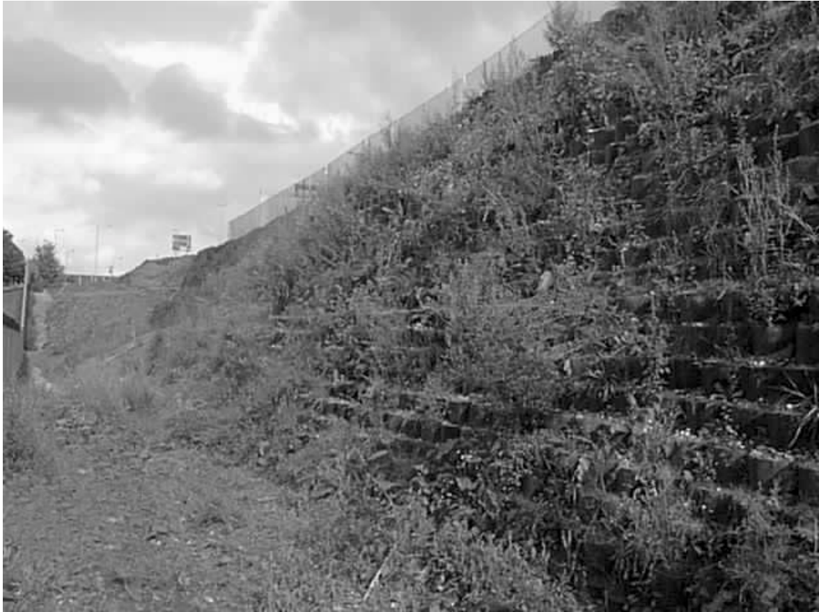
Figure 15. The same 7 m high geocell retaining wall a few weeks after construction. Natural vegetation has established itself to achieve the desired natural appearance.
