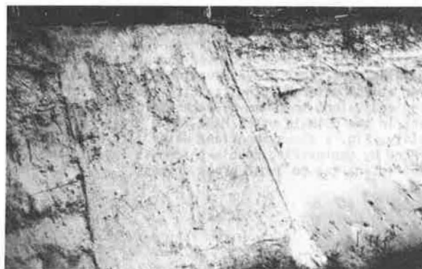
Photo 5 : On 4.4.85. Grass covering is poor and scarcely distinct on the photography. Geotextile is beginning to be destroyed at the top.
