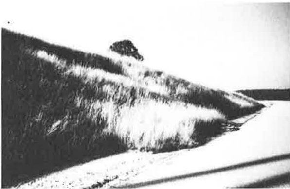
Photo 8 : Vegetal earth layer has a good vegetal covering, but is not tied to the slope and has slid.
