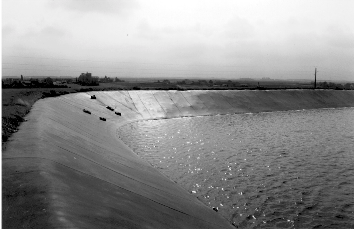
Figure 5: Préfontaine 1982 general view; note the irregular support
