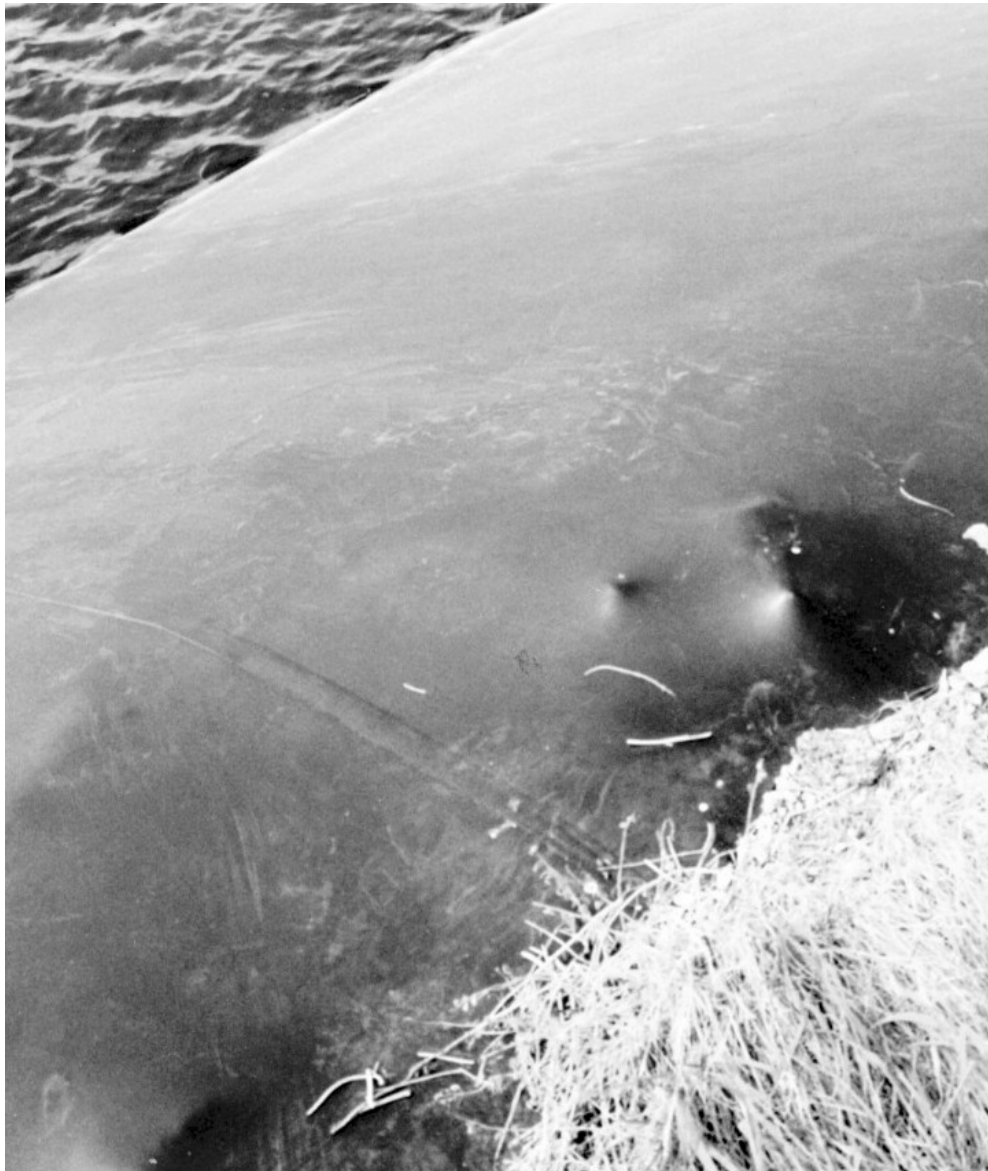
Figure 7: Préfontaine: note heavy puncturing due to stones below the geomembrane, without failure after 18 years.
