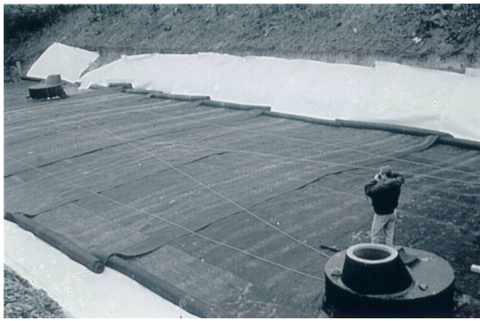
Figure 6. Installation of the upper layer of geogrid R 1200/50-10 made from aramid, Road B 180, Neckendorf near Eisleben, Germany, 1993
