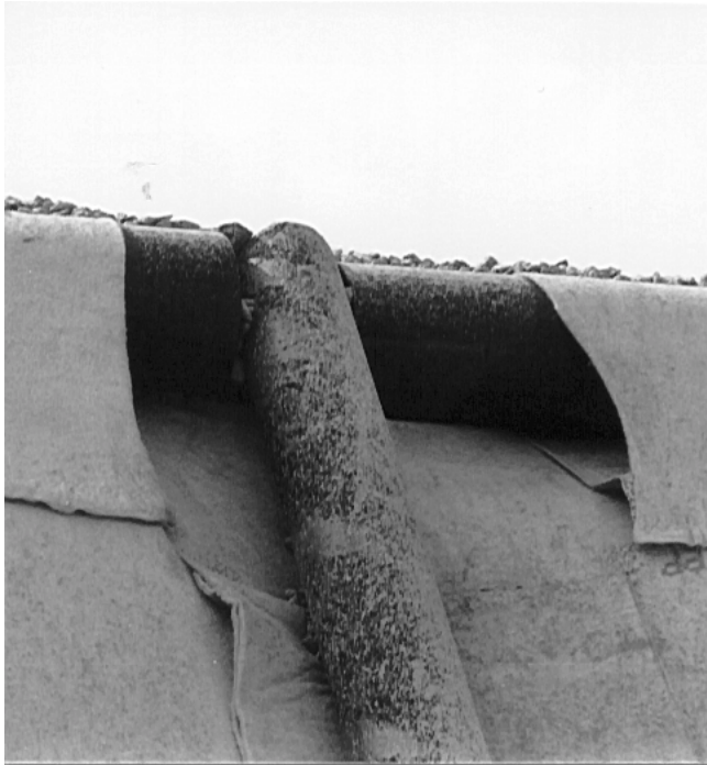
Figure 6: Open flames are used for welding nonwoven material on the upper steel tube
