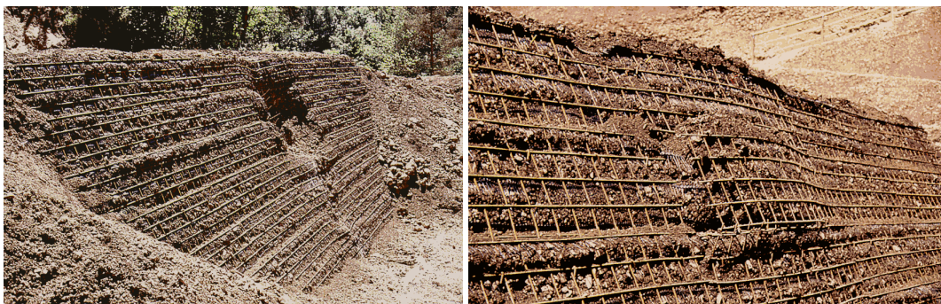
Fig. 6: Deformation of the wall due to the impact.
