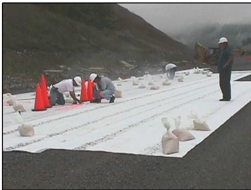
Figure 3. Installation of the geocomposite membrane in section J showing the wedding process, staggered installation is also shown.
