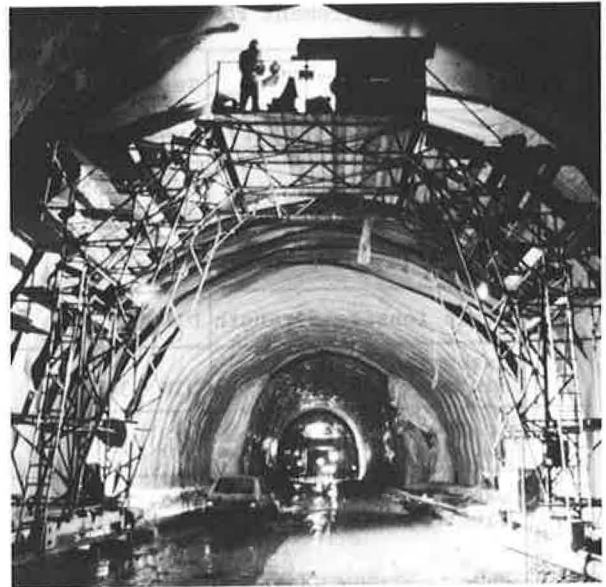
Illustration 1: waterproofing in a tunnel, by means of a protection layer and PVC-sealing boards.
