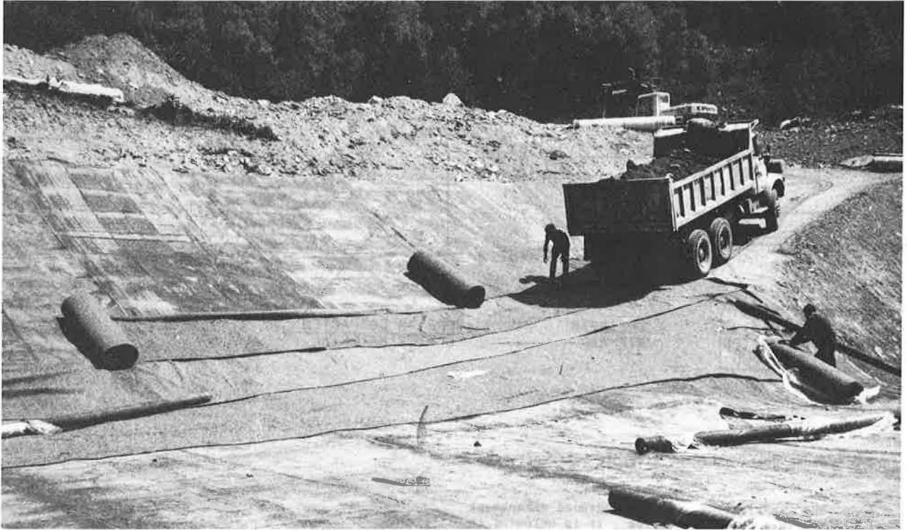
View 3 - Application of the antipunch geotextile on the geomembrane and delivery of the embankment material
