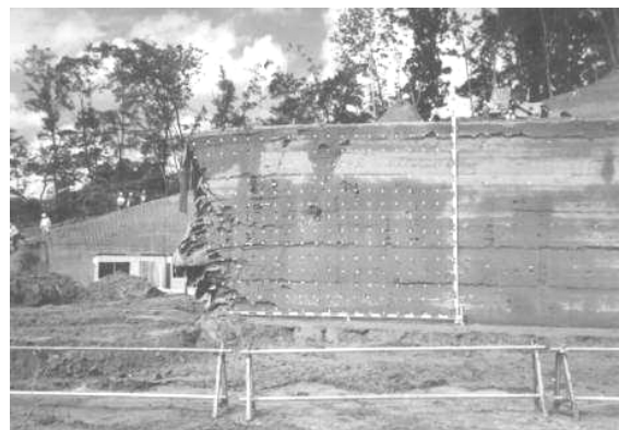
Photo 8 Falling down of the overhanging part of the reinforced fill
