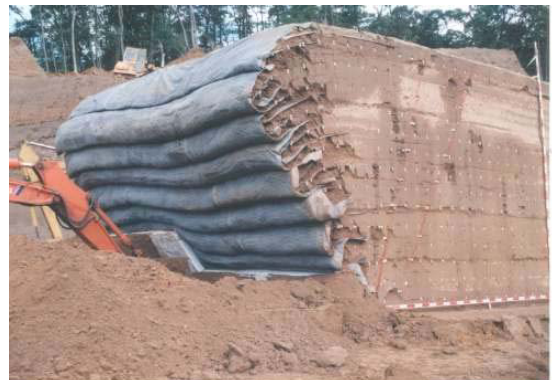
Photo 7 Excessive deformation of the third embankment in 1994
