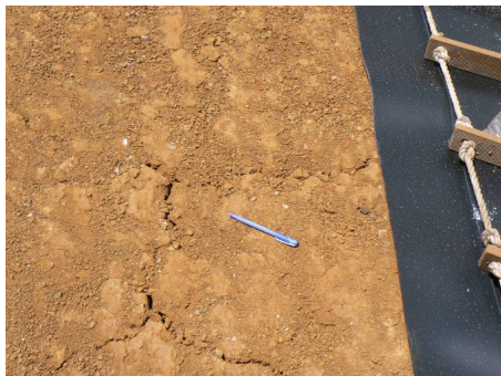
Figure 4. Photograph of a clay liner just before placement of overlying GM. Note desiccation cracks.
