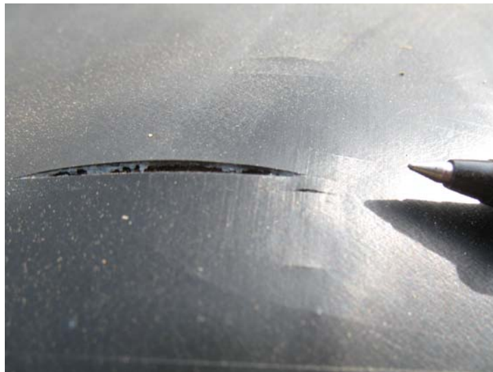
Figure 7. Stress cracking along extrusion die lines at subgrade stone protrusion.
