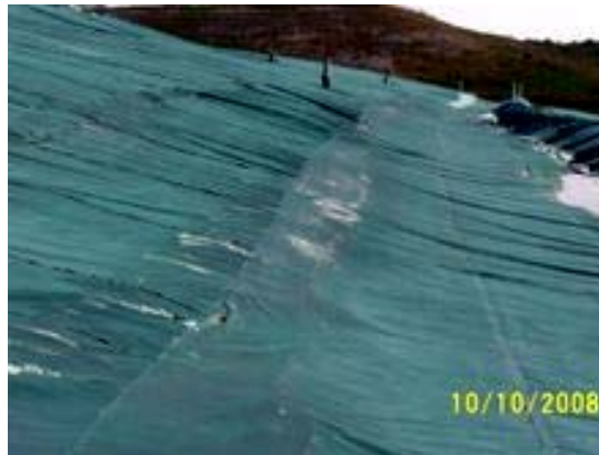
Figure 3. Exposed reinforcement (white) on sunny side (Courtesy DSWA)
