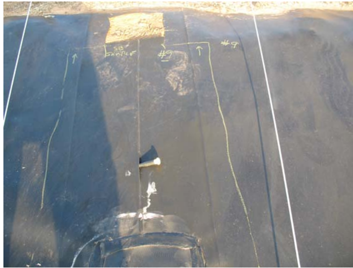
Figure 6. Stress cracking (screwdriver) along apex-down manufacturing fold. Anomalous apex-up folds (arrowed) are not cracked.
