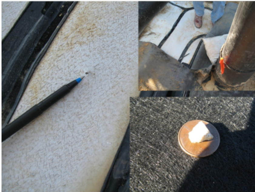
Figure 4. Small hole (at pen tip top right and left) found under 600 mm sand cover, and particle making it (bottom right).
