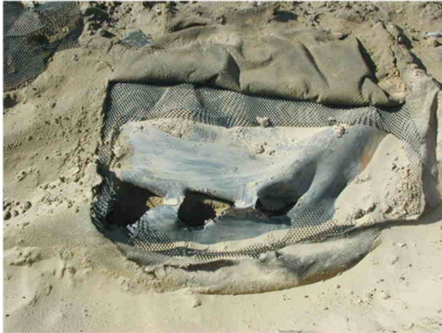
Figure 5. Typical large hole caused by mechanical equipment.
