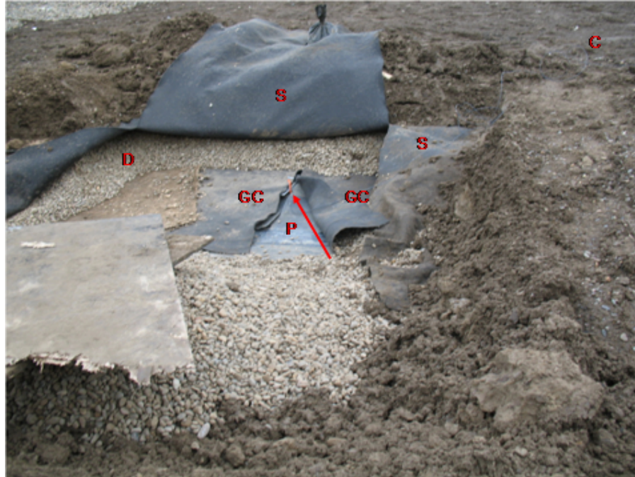
Figure 3. CRE (arrowed) attached to GCL under primary geomembrane (P). Primary geocomposite (GC), gravel drainage layer (D), separation geotextile (S), clay operations layer (C)
