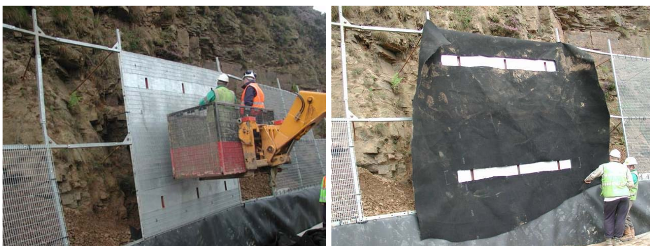
Figure 4: 4a on left shows 3m x 3m instrumentation panel being installed within revetment steepwall. Lower lift of geomembrane visible below. Vertical slots in front face for instrumentation visible. Gap in mesh shown at level of slots. 4b on right shows placement of quarry-side NPNW geotextile protection. Horizontal gaps in NPNW and mesh designed to allow movement in HDPE bars welded to rear face of the geomembrane (see text for further explanation).
