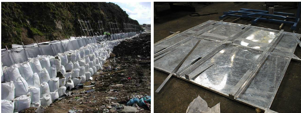
Figure 3: 3a on left is a general view of the revetment system showing bulk sacks and waste in front of steepwall. 3b on right is a rear view of instrumentation panel prior to installation. Three SHS are shown welded to rear face with access slots for installation of the transducers from rear. 'Top' of panel shown in foreground of image.
