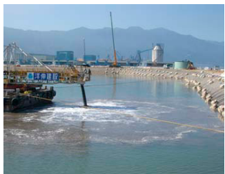
Figure 11. Discharging slag by FCS
