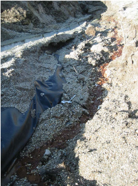
Figure 3 Leachate percolation along the landfill cover.
