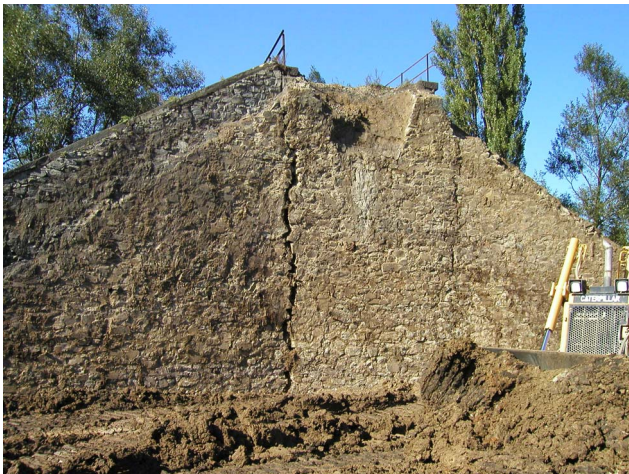
Figure 3 Vertical cracks separating wing walls and bridge abutment (inner side)
