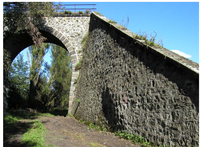
Figure 2 Deformed wing wall
