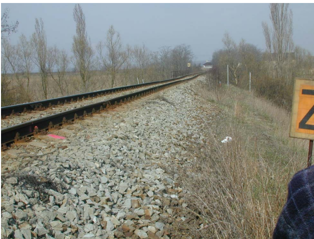
Figure 1 Deformed rail track near the bridge
