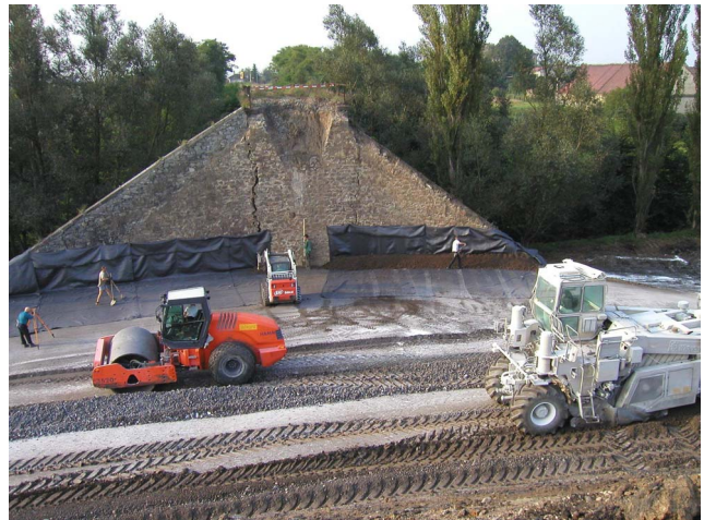
Figure 7 General view of the site during the stabilisation and soil reinforcing works
