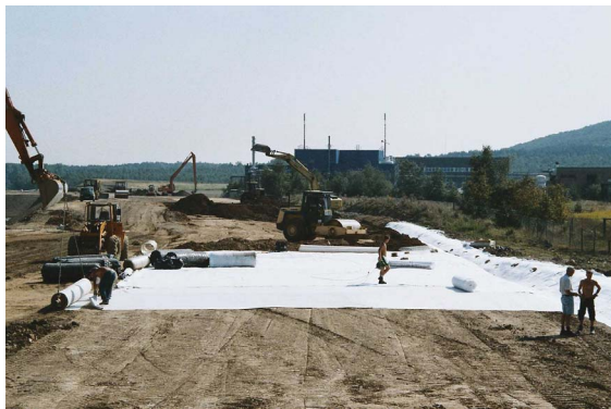
Fig. 6: Installation of geosynthetics in the infrastructure sealing application by-pass road B 82n Langelshheim, Germany
