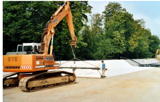
Fig. 5: Installation of the needle-punched geosynthetic clay liner serving as RiStWag sealing in the project B 3 Wasser near Freiburg
