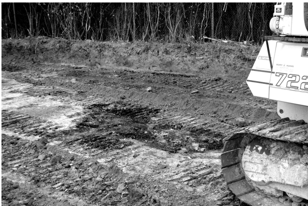
Figure 2 Area of organic waste with dark colour after removal of the soil cover
