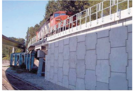
Figure 7. MSE wall supports heavy rail load in Vancouver, Canada.
