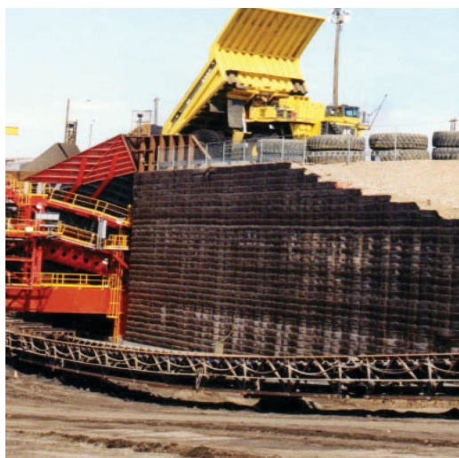
Figure 3. Heavy hauler mining truck dumps into hopper/crusher while supported by bar mesh temporary MSE wall.
