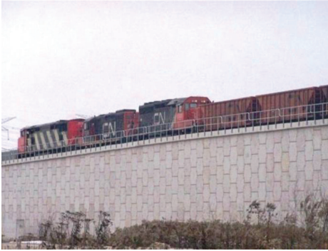
Figure 8. Heavy rail load on MSE wall in Toronto, Canada (Design load of Cooper E90).
