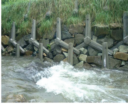
(a) Flood condition of revetment at Yamaguchi City
