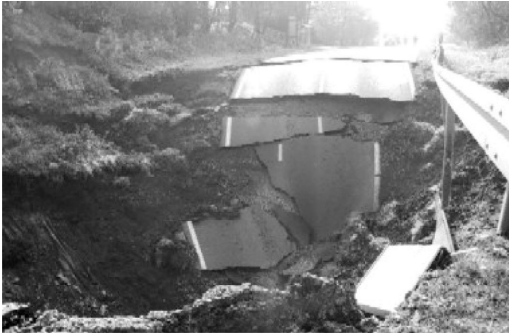
Figure 8. View in the morning after the renewed sinkhole activity.
