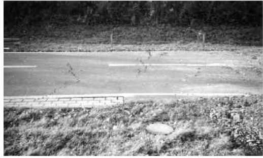
Figure 9. Cracks in the asphalt in the geogrid-anchorage zone; the funnel is to the right, just out of the photograph; one of the control chambers in front.
