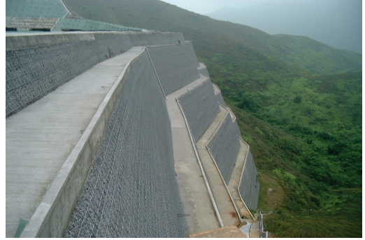
Figure 7. Completed reinforced fill embankment on the side facing away from the waste.
