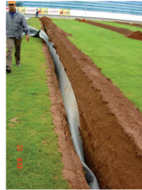
Photo 1. During the construction of the trenches and insert of the geocomposite drain.
