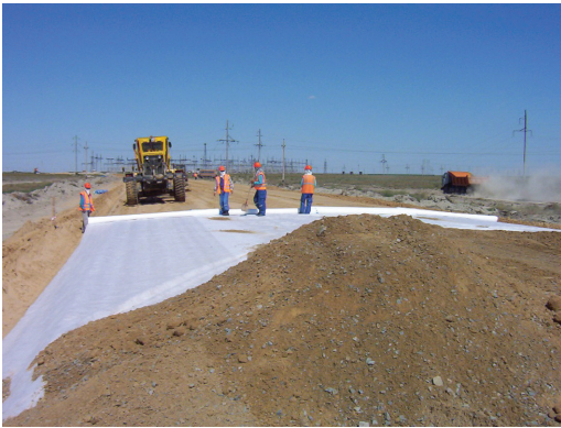
Figure 7. Installation of reinforced soil of “The new western road” object (Atyrau city, Kazakhstan, 2003).
