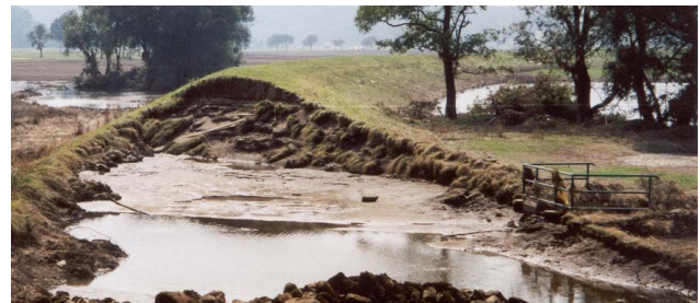
Figure 2 Mulde River dyke failure in August 2002
