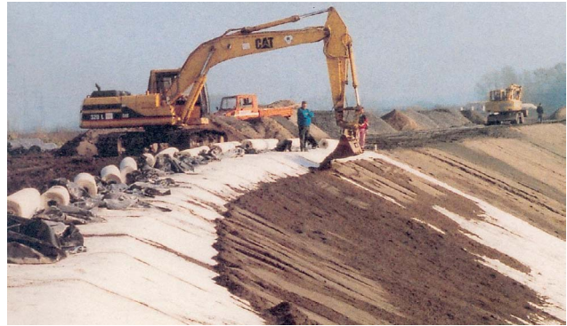
Figure 9 Installation of a GCL for use as dyke sealing system on both Lippe River sides near Haltern-Lippramsdorf and Marl (1994)
