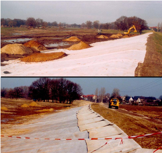
Figure 8 Mulde River dyke already protected during the construction phase: Installation of GCL on the slope at the water exposed side 2002 (top); already swollen but intact GCL which has been folded back to be able to drive on the dyke crown after the flood in winter 2003 (below).
