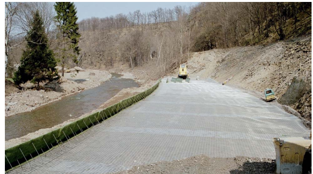
Figure 11 Installation of geogrids as reinforcing as part of flood railway rehabilitation in Weesenstein (2002)
