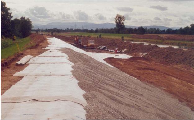
Figure 5 Reconstruction of the Kinzig River dyke in 2001 - installation of non-cohesive cover soil from the river bed
