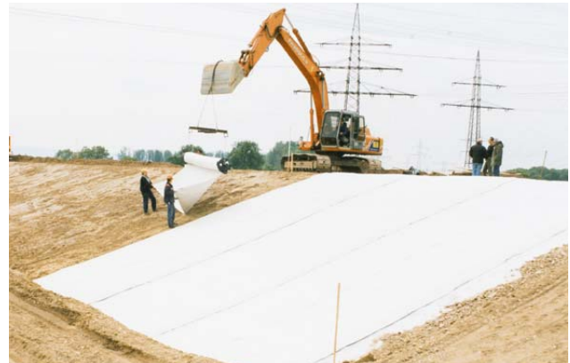
Figure 4 Reconstruction of the Kinzig River dyke in 2001 - Installation of GCL Bentofix® B4000 (installation by means of a spreader bar)
