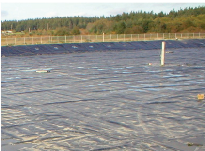
Figure 1. Wrinkles in the HDPE geomembrane at the end of installation.
