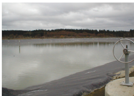
Figure 3. Removal of the “bubbles” has completed the installation and start-up process for the lagoon.
