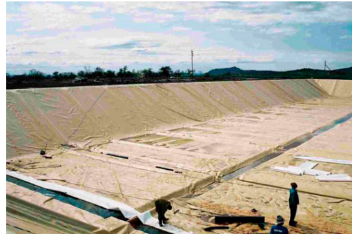
Plate 6: The molasses reservoir during commissioning
