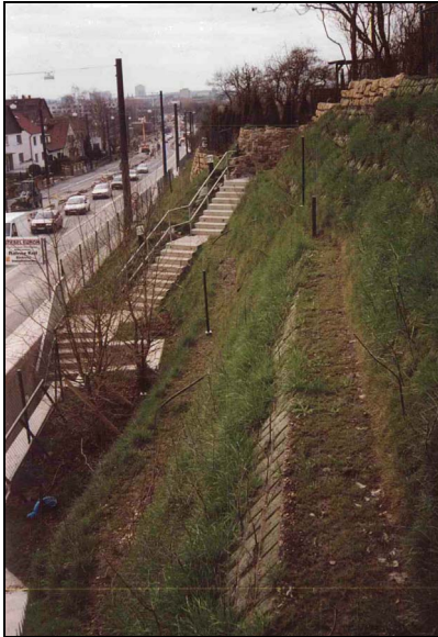
Figure 14: GRE-Erfurt Galgenberghang/at date of commissioning
