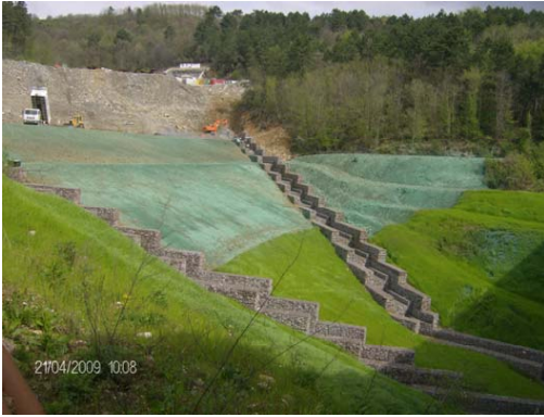
Fig. 12 – The reinforced embankment and the gabion channel during construction: the bottom part is already vegetated, the upper part has just been hydroseeded
