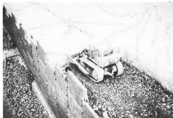
Fig. 1 Jersey wall under construction. Rock fill being placed over Paraweb and Terram
