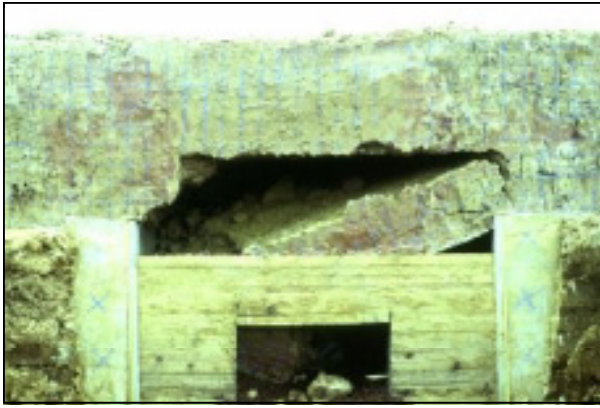
Figure 6. Collapse of the lower sub-layer of the unreinforced earthwork during emptying.
