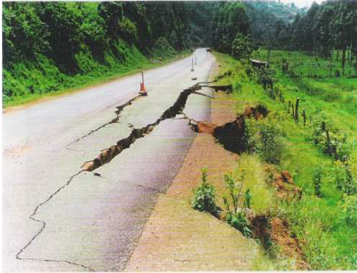
Figure 20. Deep tension cracks in surfacing.
