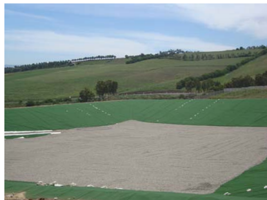
Figure 38. Geocomposite on side wall and granular drainage layer at the bottom of the cell
