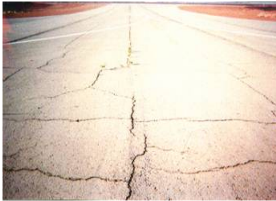
Figure 24. Transversal cracks due to thermal stresses
