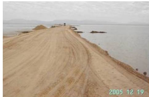
Figure 16. View of the partially inundated pilot road route test (prior to reinforcement solution).
