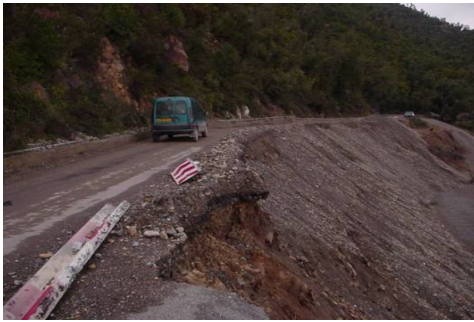
Figure 7. View of the damaged road and slope failure
