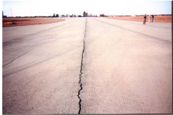
Figure 25. Longitudinal cracks along the asphalt strip joint
