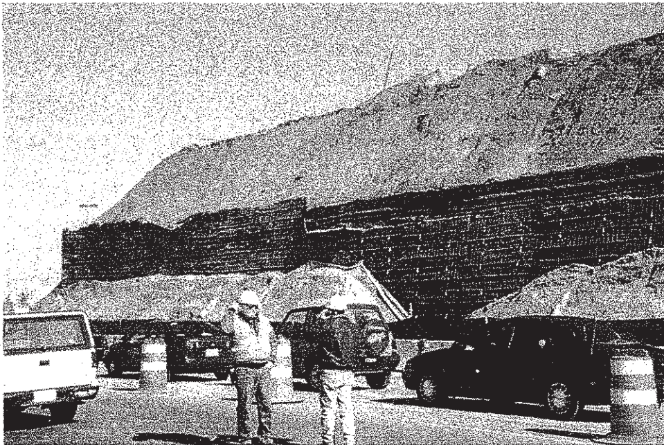
Figure 4. Temporary surcharge on wirewall, Atlantic City.
