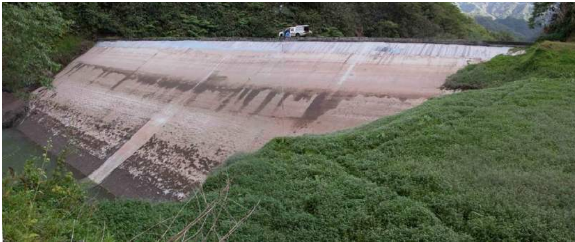
Figure 4. Typical dam in Tahiti; 1.0 mm PVC-P Geomembrane
