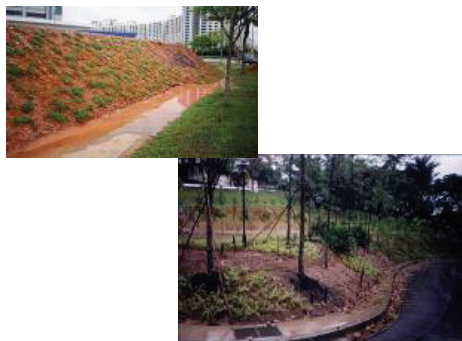
Figure 1. Examples of urban road side construction with serious erosion and sediment concerns
