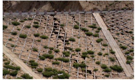
Figure 3. Slope erosion disables the slope protection.
