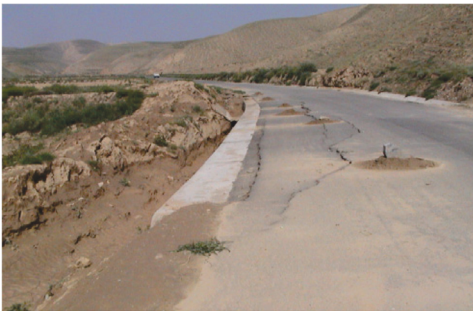
Figure 1. Longitudinal crack on pavement.
