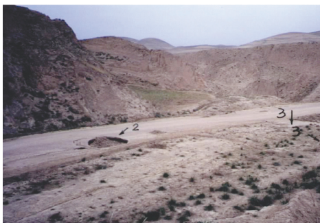
Figure 2. Roadbed cavity on Line Xiji-Haiyuan Highway.
