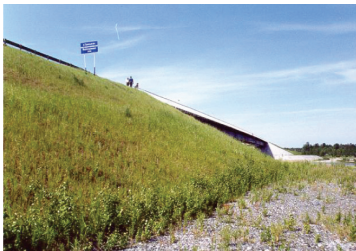
Figure 3. General view of bridge approach slopes across the Tromyegan river. Slopes are reinforced with geocell (Surgut – Nizhnevartovsk road, Hanty-Mansiysk autonomous region).
