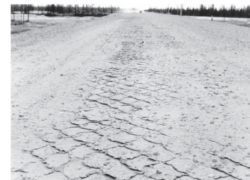
Figure 6. Damaged pavement section of Tarko-Sale road, Yamalo-Nenetsk autonomous region.
