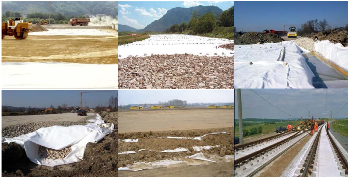
Figure 1. Some applications of needle-punched non-woven geotextile on road and railway construction
