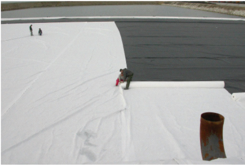
Figure 2. HDPE geomembranes (about 7 m width) are protected by a geotextile (contractor Imperfaglia).
